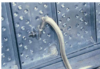
Example of earthing
